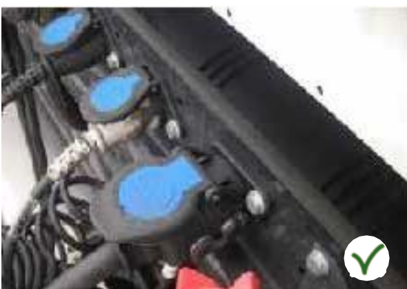
Air lines and cables are in the right place.
