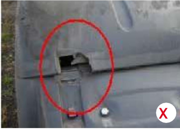
Tab and cover damaged
