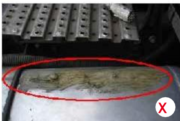
Improper repair of the tank with sealing compound or similar.
