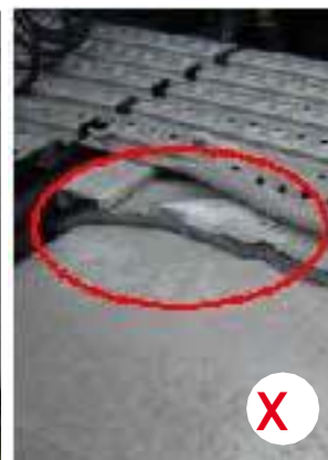
Damaged bracket and walkway
